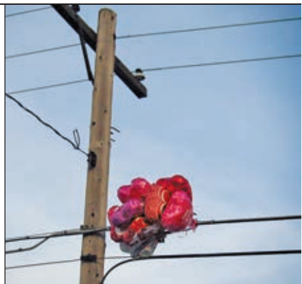
Valentine balloons and power lines are likely to create an unromantic outage.
