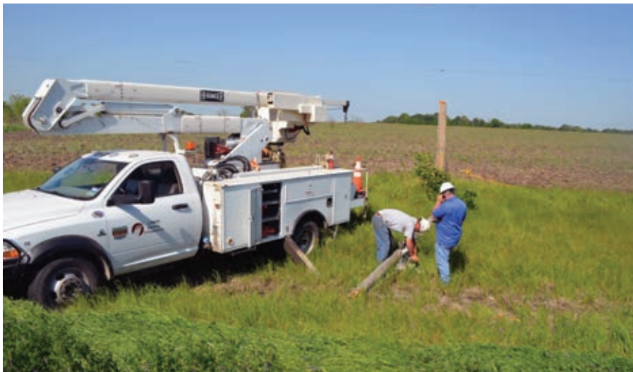
Drew Conder and George Scroggins pick up a pole that had been hit by a tractor.
