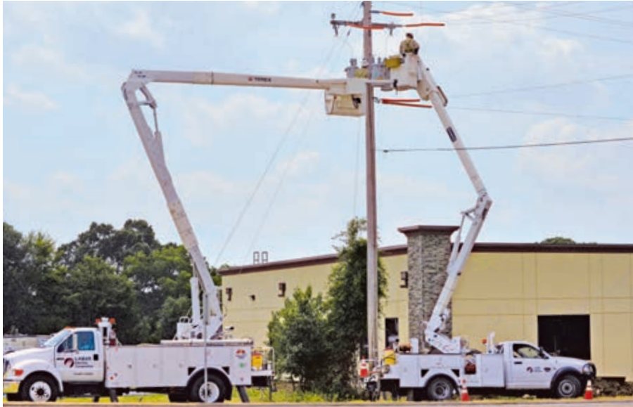
Charles Brazeal and Cory May install transformers to provide power to the new dental office.
