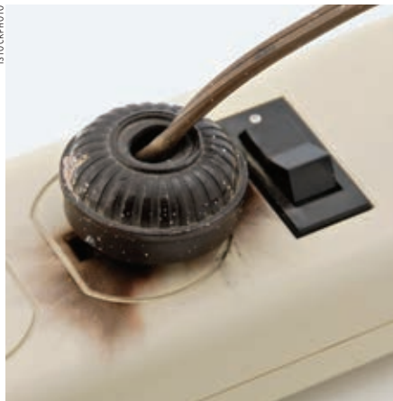
Any discoloration around an electrical outlet requires immediate attention and repair.
