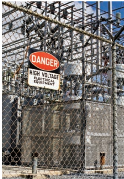
Thieves in substations are not just risking getting caught, they're risking their lives.
